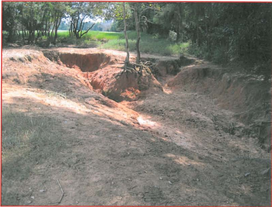
FIGURE 3D: VIEW OF SIGNIFICANT EROSION (FACING SOUTH)
